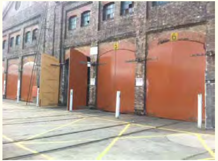
Some of the new large access doors recently installed at the Large Erecting Shop as part of the upgrade works. Photo: Keith Audet
